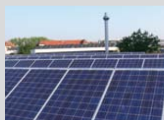
Solar-Uni Freiburg, Germany, 550 kWp
